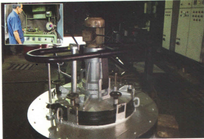
Heat Treatment Plant
